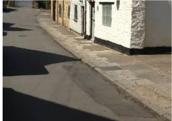
Poorly maintained roads and pavements and use of concrete kerbs and paving slabs
